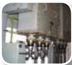
Power sensitive equipment
